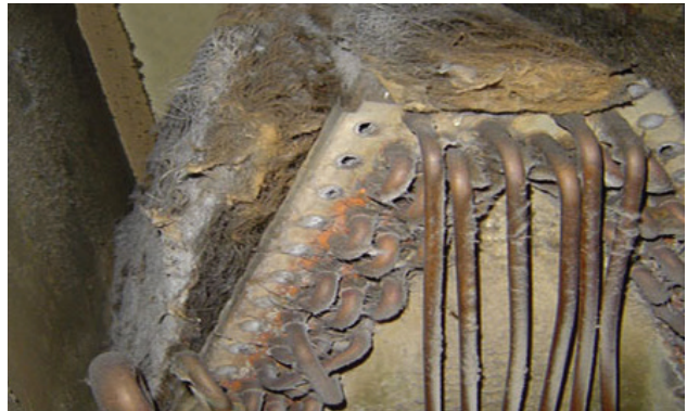
Dirty and frozen indoor AC coil resulting from the use of a standard one inch filter and improper replacement schedule.
