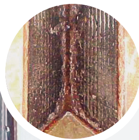
Indoor A-coil in a 10-year-old HVAC system that used a one inch filter
