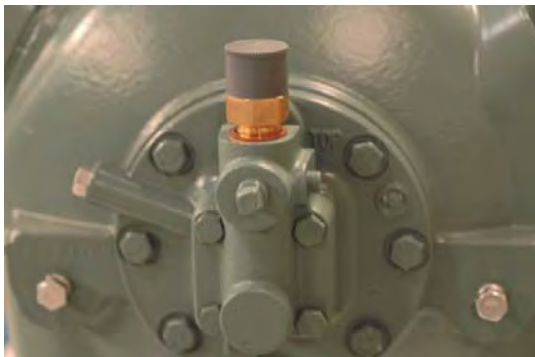
Fig. 20 — OPSS Sensor Installed
