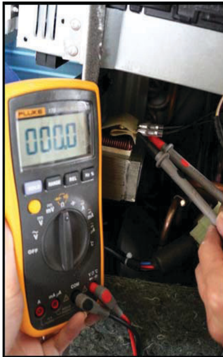
Fig. 24 —Test the Reactor resistance
